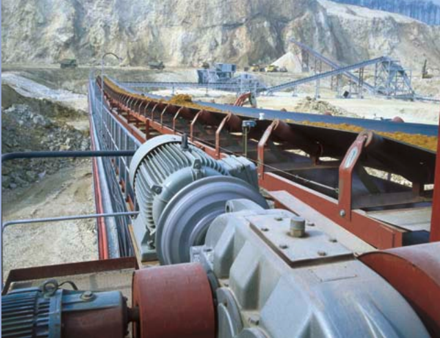
Fig. 25: Voith Turbo fluid coupling in a belt conveyor drive
