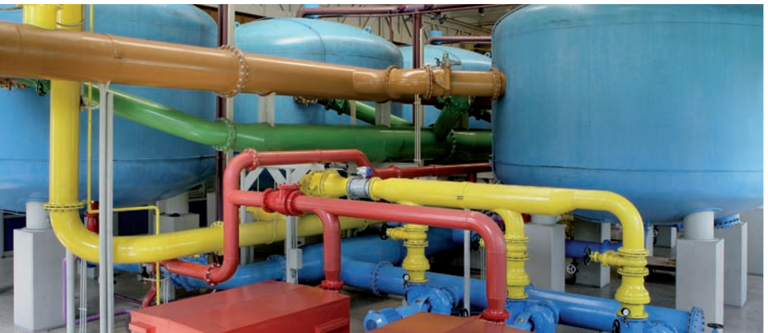
Turbidity measurement for filter monitoring
