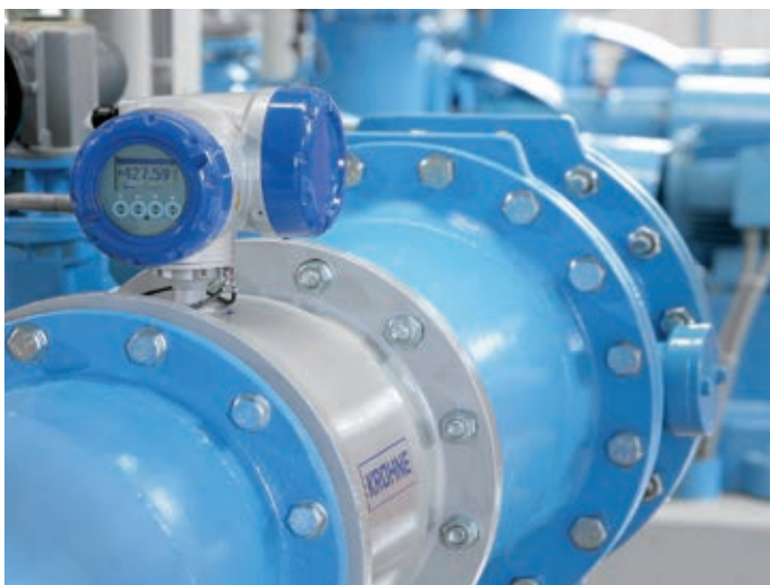
OPTIFLUX 4300 in the filtration system in city waterworks
