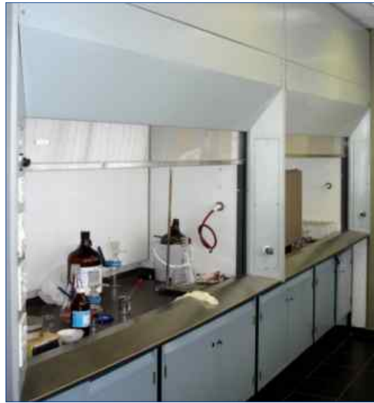
A typical Constaflow fume cupboard installation.
