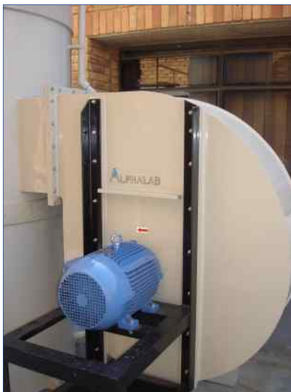
A typical fume extraction fan
