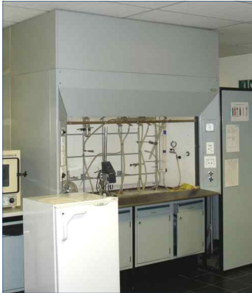
Constaflow fume cupboard.
