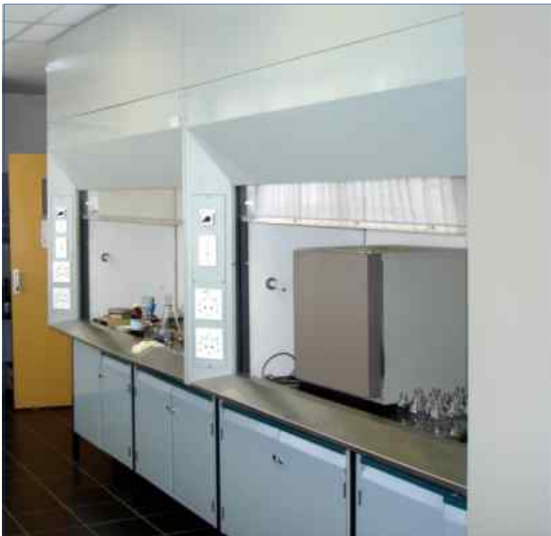
Constaflow fume cupboard.
